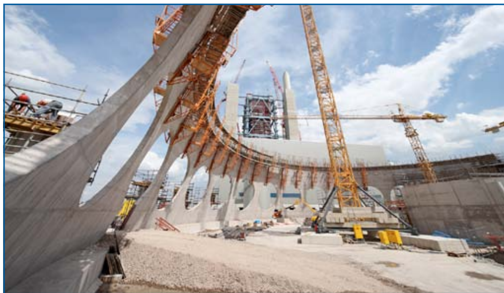
Karlsruhe Thermal Power Station (Germany)
