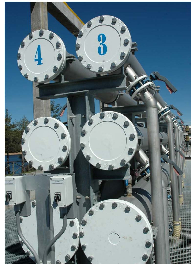
Hollow fibre membranes.
