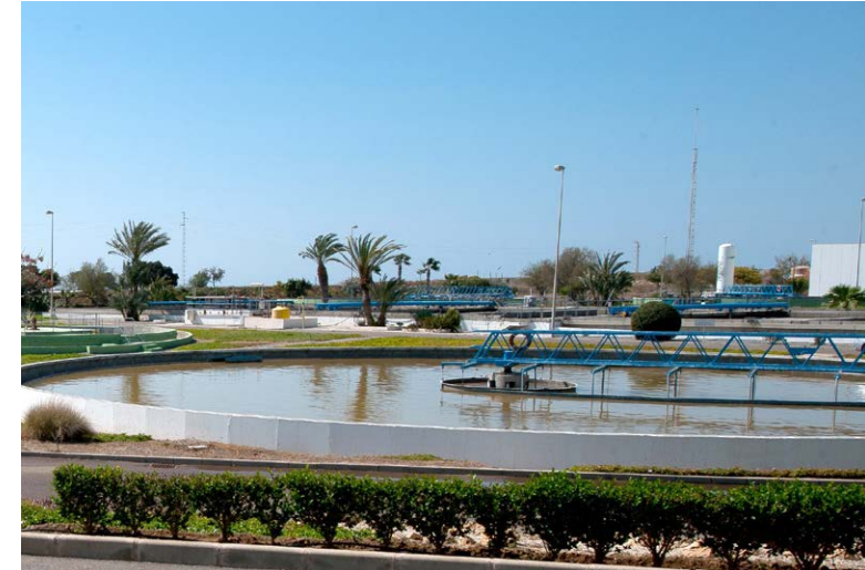
Waste water treatment plant in Almeria (Spain).
