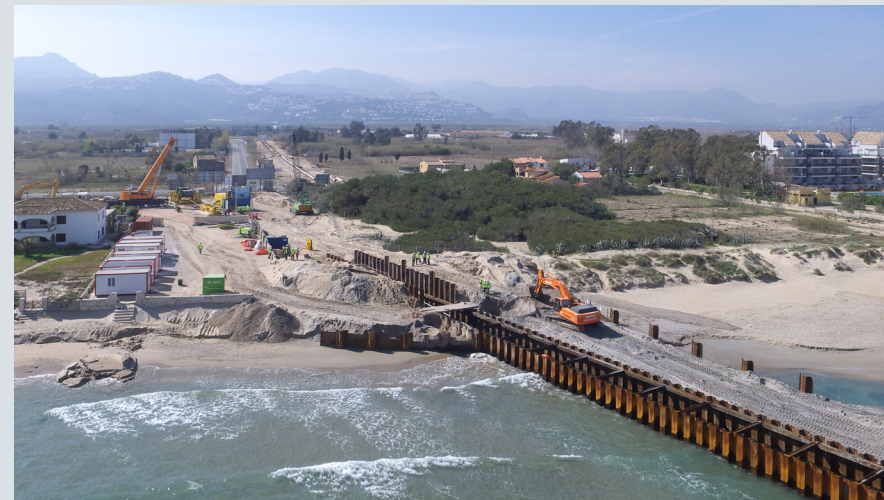
Denia Landfall 3. Underwater gas pipeline
