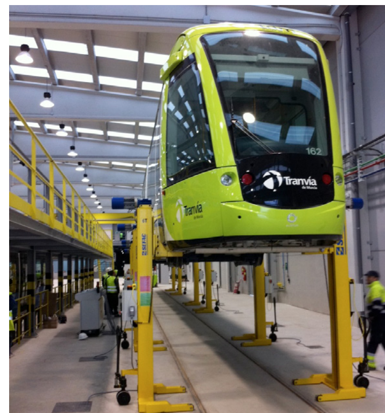
Tram maintenance facility
