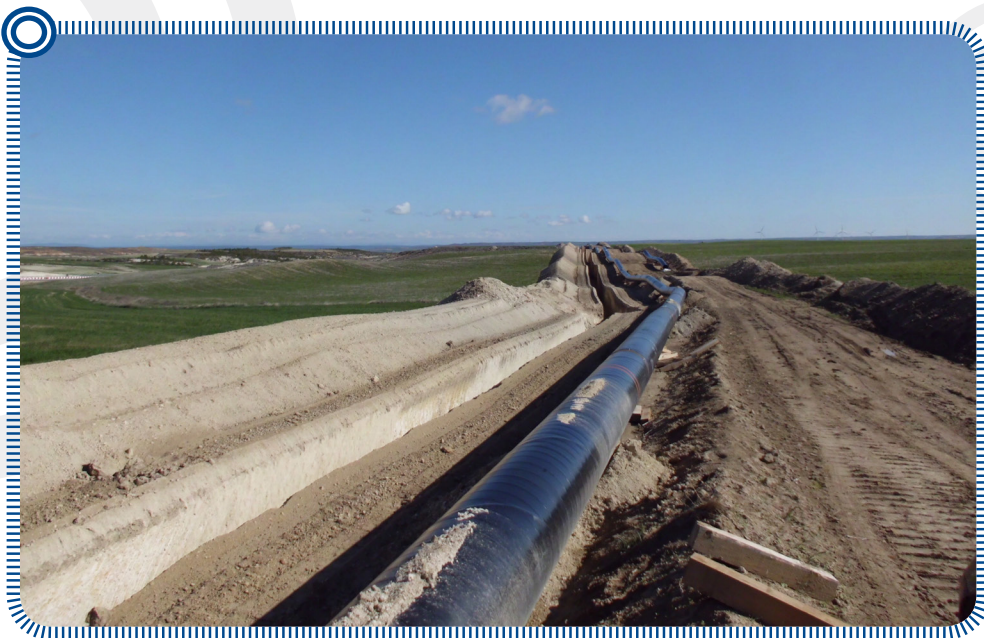
Yela-Villar de Arnedo oil pipeline.
