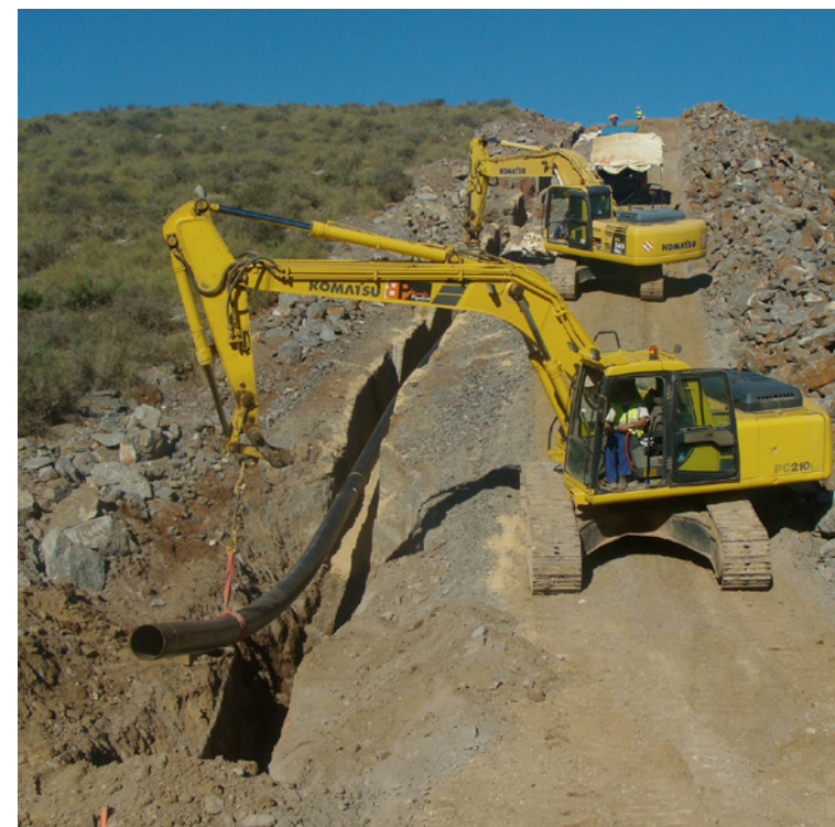
Alhama/Murcia oil pipeline
