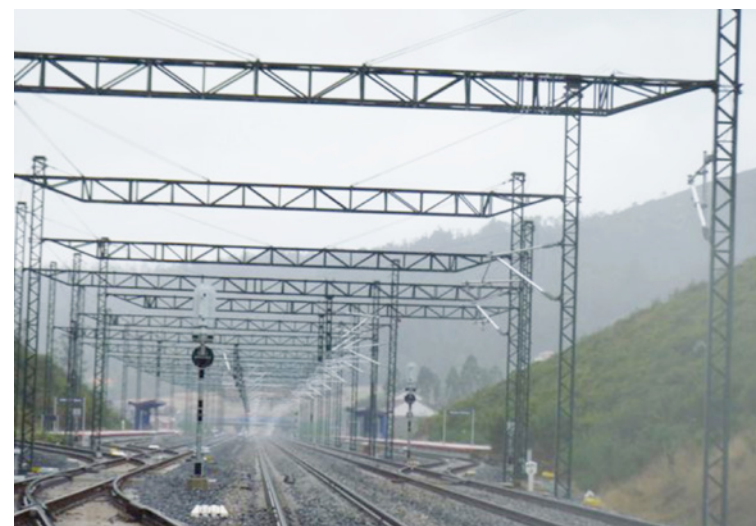
Catenary on the high-speed Atlantic Artery
