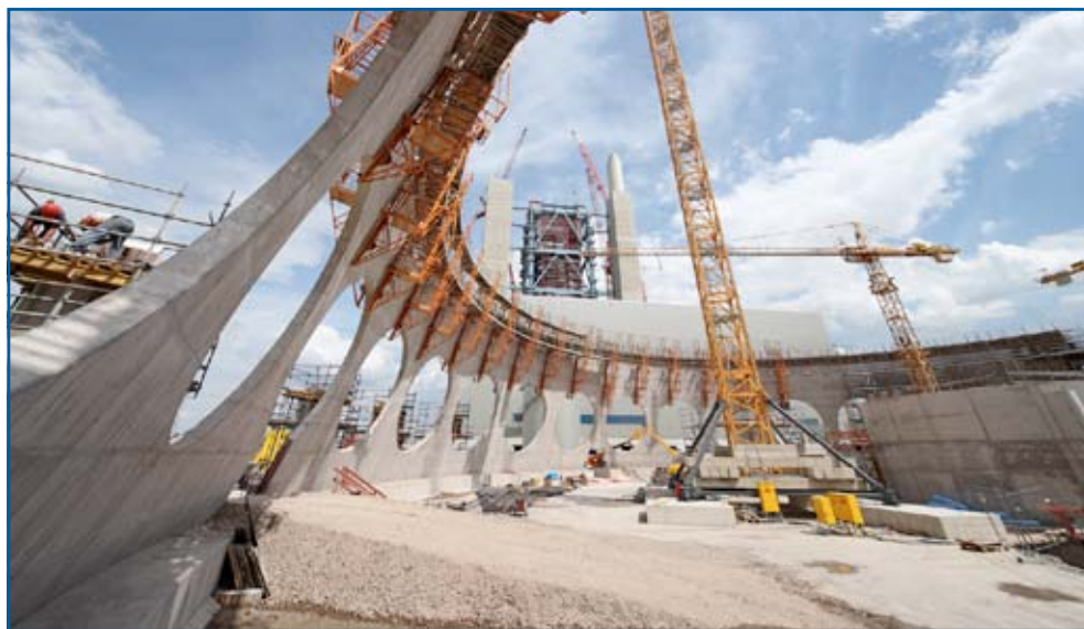
Karlsruhe Thermal Power Station (Germany)
