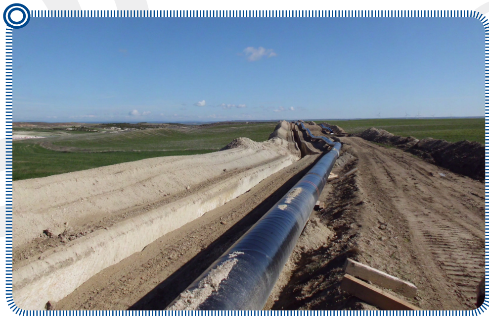
Yela-Villar de Arnedo oil pipeline.
