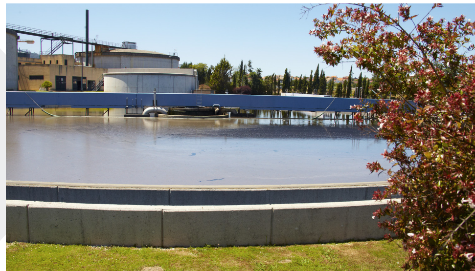
Vigo Wastewater Treatment Plant (Spain).
