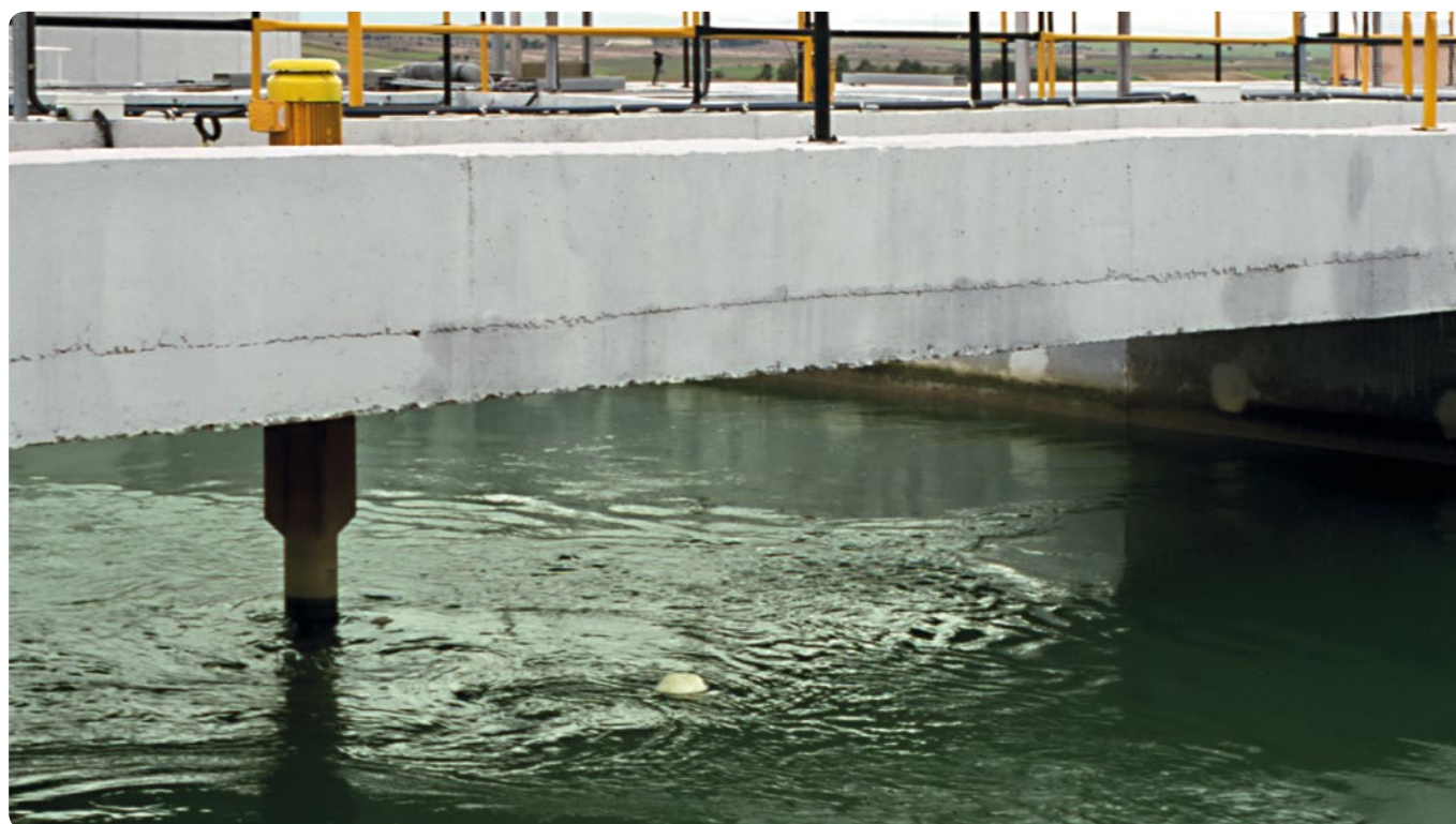
DRINKING-WATER TREATMENT PLANT, VALMOJADO, TOLEDO.
