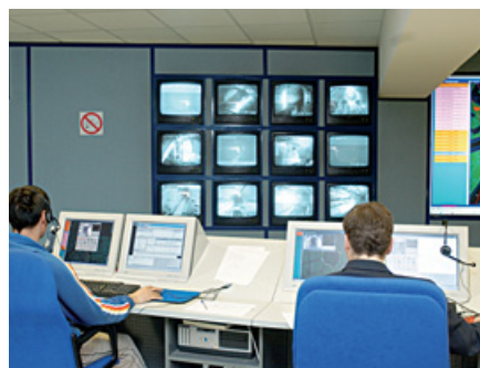
Service tunnel control centre. Madrid
