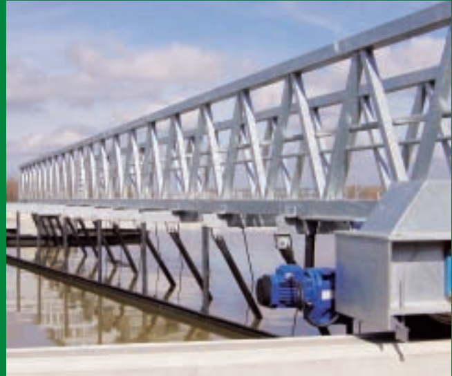
Wastewater treatment plant. Salamanca
