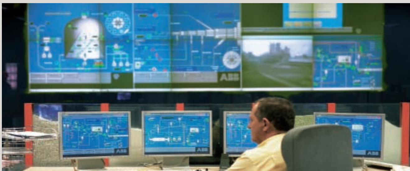
Control room of the factory at El Alto. Madrid
