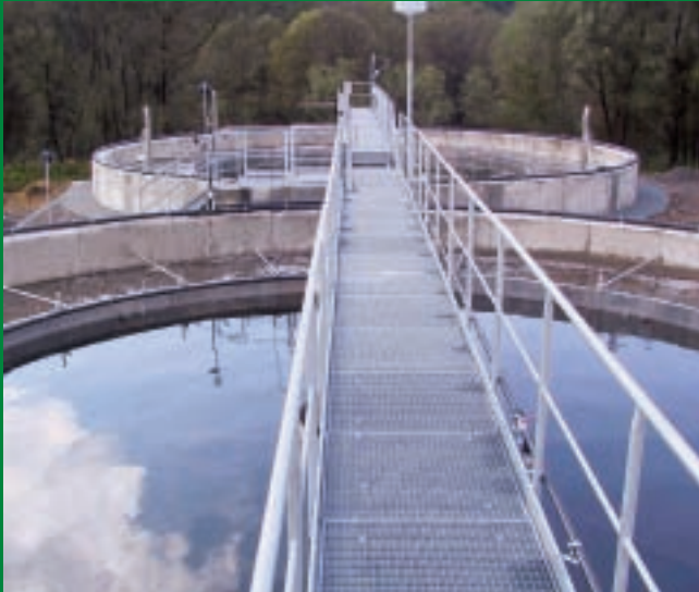
Jablunkov wastewater treatment plant. Czech Republic
