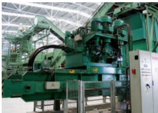
Solid urban waste treatment plant. Tudela. Navarra
