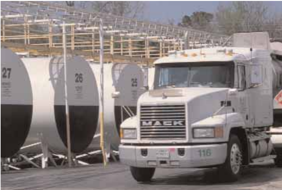
Wastewater treatment plant in South Carolina. USA.
