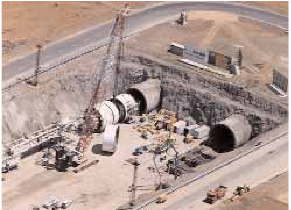
■ Guadarrama tunnels. Madrid
