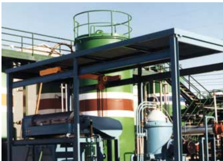
Industrial wastewater treatment plant in Valdebebas. Madrid
