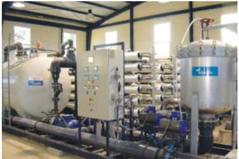
Desalination plant in Dénia. Alicante
