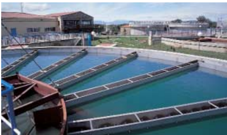
Drinking water treatment plant. Ávila
