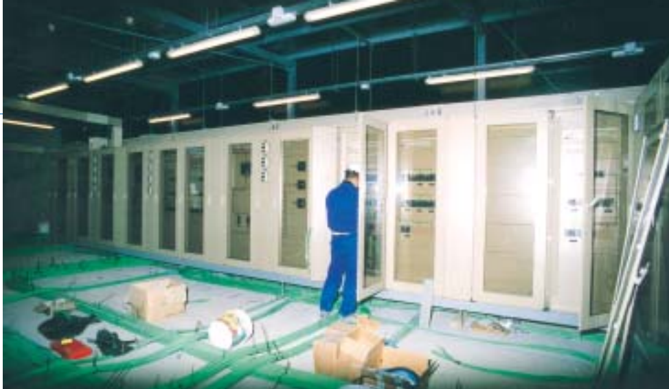
Electrical installations at the Sogecable building. Madrid.
