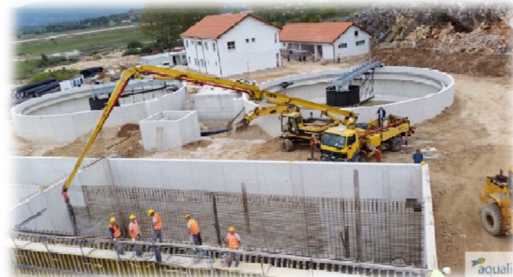
Waste water treatment plant (Montenegro)
