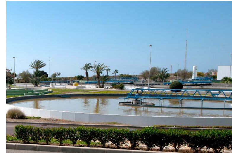
Waste water treatment plant in Almeria (Spain).
