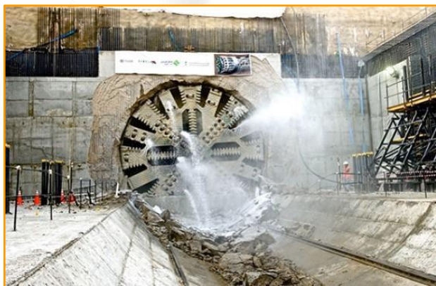
Electro-mechanical installations on lines 4,5 and 6 Riyadh Metro: €179 M
