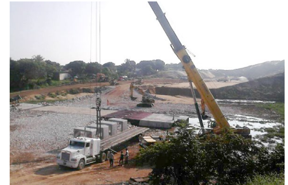
Installation of prefabricated caissons inside the lagoons in order to give continuity to water and aquatic species.
