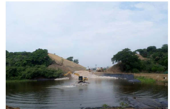
Formation of the embankment by fragments of rock with different sizes and weights.
