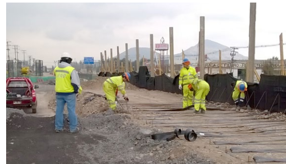
Use of steel slag in the core of the embankment for one of the walls.
