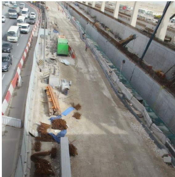
Construction of the motorway underpass in the northern area of the project.
