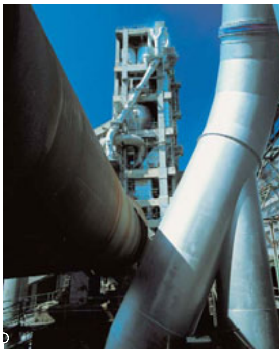
THIS PRACTICE IS DEVELOPED IN THE CEMENTOS PORTLAND VALDERRIVAS factory at Lemona, where, in addition to used tyres, the company uses recycled plastics, wood, or animal meal.
